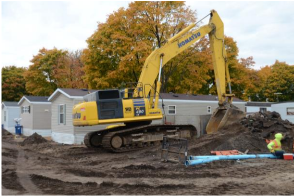
Park Plaza Cooperative in Fridley, Minn, spent millions to replace its water system and repave roads.
